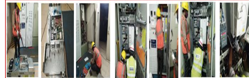
Unit-1 LT Drives Preventive Maintenance Activities Pic
