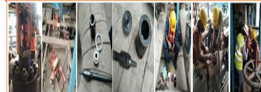
Control Valve Dismantling, Gasket Replacement, stem, seat, cage, aping, blue matching & calibration
